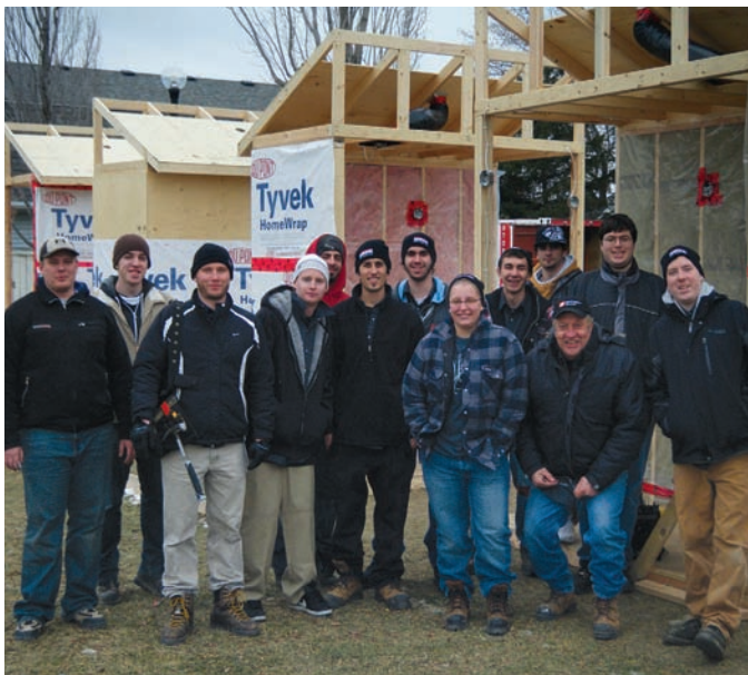
Niagara Peninsula Homes' Rick Sherk (centre), the program supervisor of Team ENERGI Program 2, is alongside the 12 program participants at Commonwealth Cooperative Homes in St. Catharines following the completion of the working component of the 6 month work experience program.
