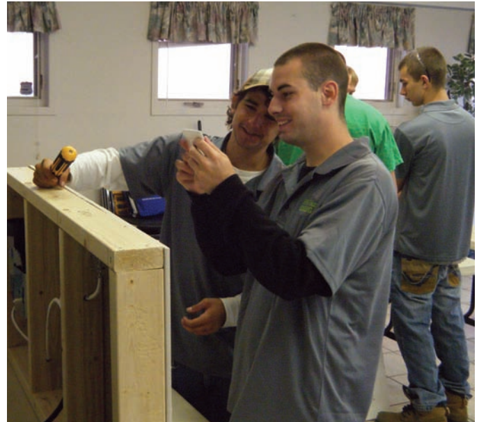
Jacob Good and Ray Catton of Niagara Peninsula Homes’ Team ENERGI Program 1 work together at Meadowgreen Cooperative Homes in St. Catharines to learn new skills, while under the direction of program supervisors and trades people.
